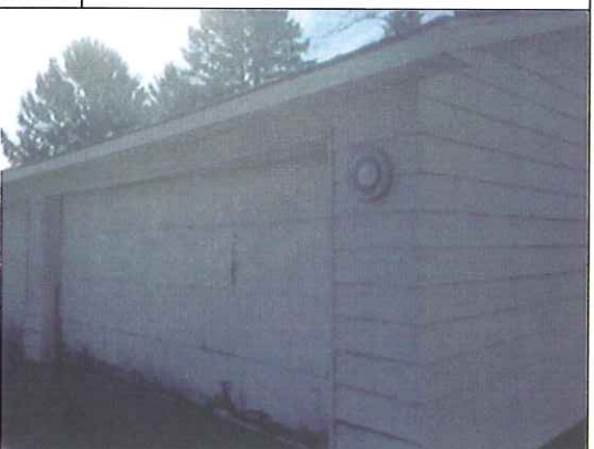
Photo # 11: Garage Exterior, Roof Shingle Layers
