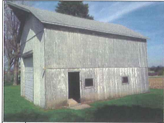
Photo # 14: Barn, Exterior Roof Shingle Layers, Window Glazing, and Door Caulk
