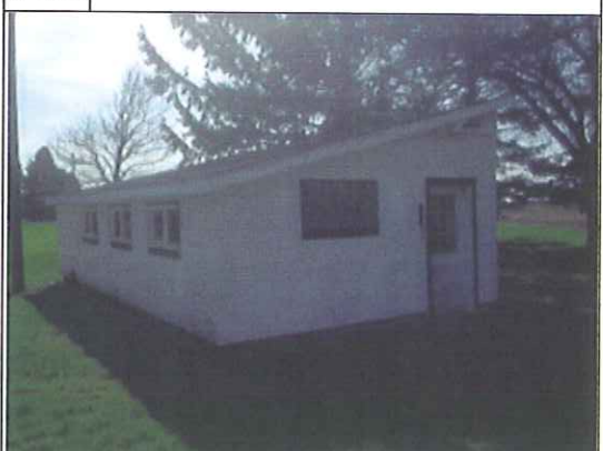
Photo # 12: Southeast Workshop, Exterior Roof Shingle Layers, Window Glazing, and Interior Drywall/Mud/Tape
