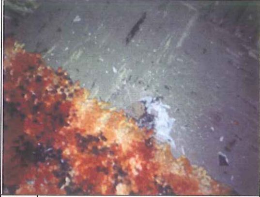
Photo #7: House Interior, 9" x 9" Gray Vinyl Floor Tile and Mastic (2 nd Floor)
