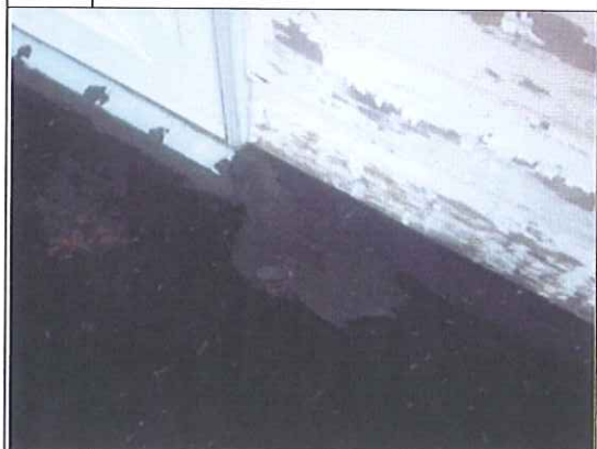
Photo # 10: House Exterior, Roof Tar
