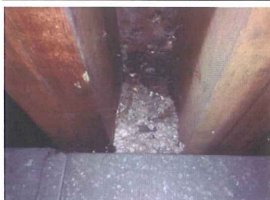
Photo #6: House Interior, Plaster (in Basement Walls)
