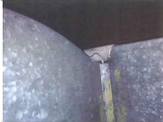
Photo #4: House Interior, Duct Tape (Mainly Basement)
