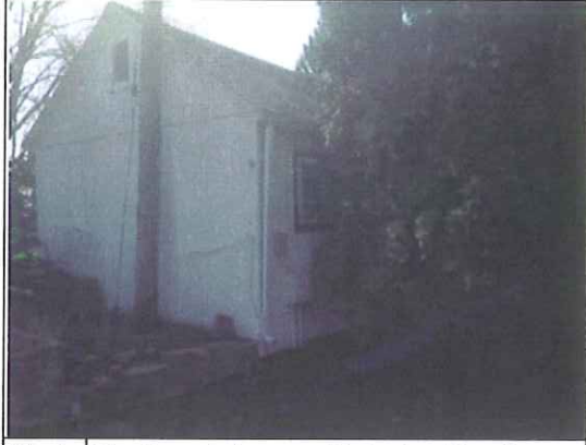
Photo # 13 Northeast Annex, Exterior Roof Shingle Layers and Interior Drywall/Mud/ Tape
