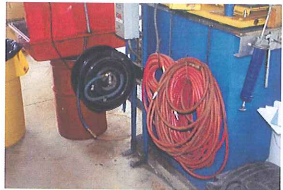
Hoses and cords off the floor
