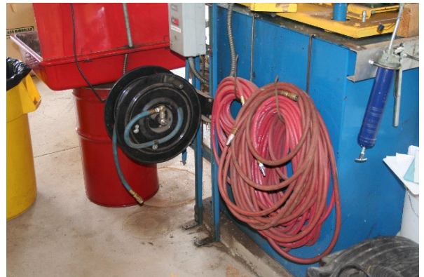
Hoses and cords off the floor
