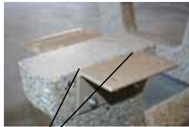
Make sure angles are not misaligned as shown.
