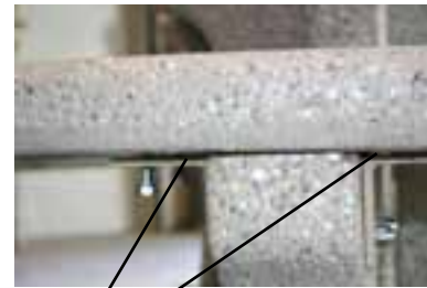
Angles are below concrete legs. Not aligned properly.
