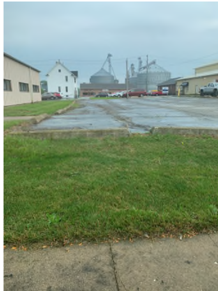
Deteriorated parking lot South of 520 N Maple St
