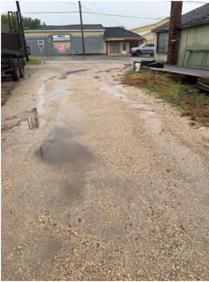
Deteriorated right of way near 418 N Main St
