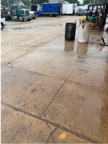
Cracked and deteriorating pavement at 416 N Main St
