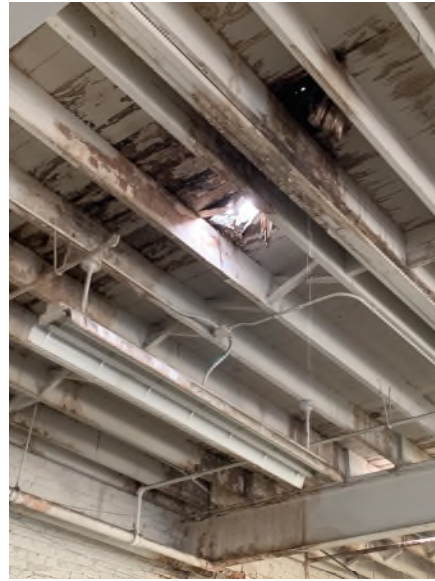
Dilapidated and deteriorated roof leaking water at 433 N California 2
