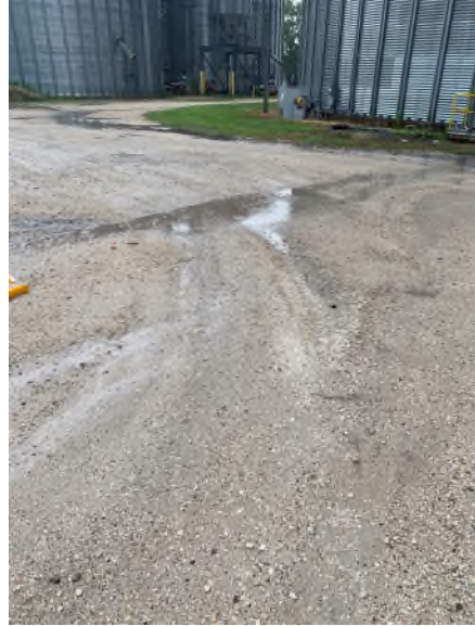
Deteriorated drive near 418 N Main St
