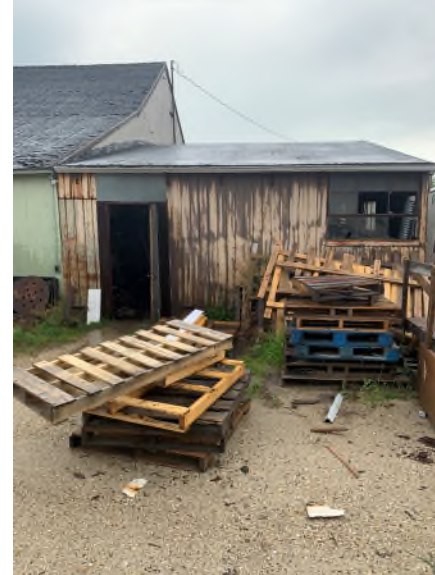
Missing window panes and deteriorated siding at 418 N Main St
