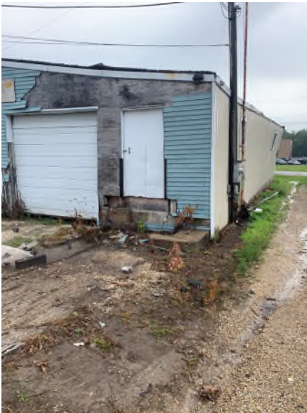
Dilapidated and deteriorated siding, wall, and roof at 426 N Main St
