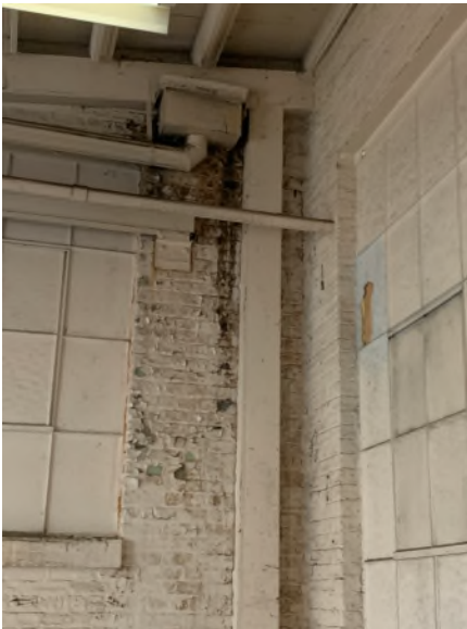
Deteriorated interior wall with water damage at 433 N California St
