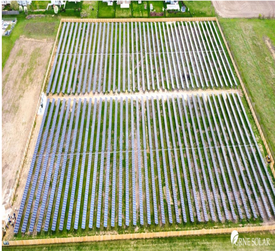
Kendall County, IL (Public Safety Building, Courthouse and Health Services) Annual Production = 3.3 million kWh/year Lifetime Production = 82.5 million kWh's
